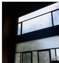
BEL Replace fogged window panes
