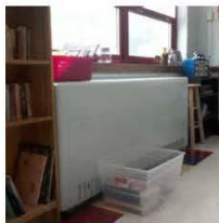
BEL Replace through-wall heating units
