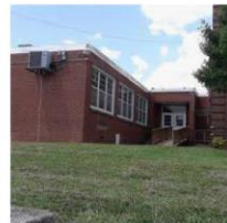
SMS Replace handicap ramp at front
